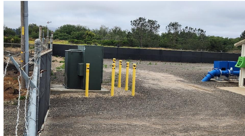
Photograph 6. Pad-mounted transformer inside fenced well enclosure in eastern portion of subject property
