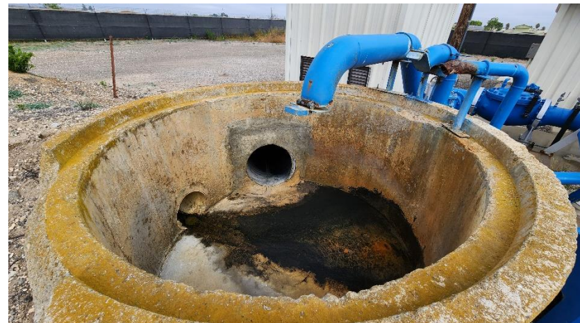
Photograph 4. Discharge basin for flushing the well, connected to stormwater system in eastern portion of subject property
