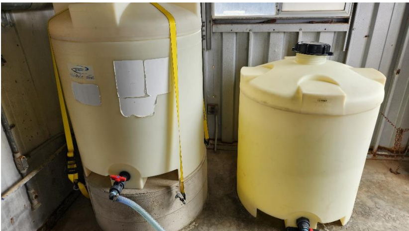
Photograph 3. 100-gallon chlorine tanks in well pump housing in eastern portion of subject property
