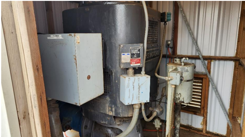
Photograph 5. Well pump in housing on eastern portion of subject property
