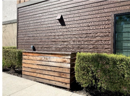
Screened mechanical equipment and vents painted the same color as the adjacent building facade.
