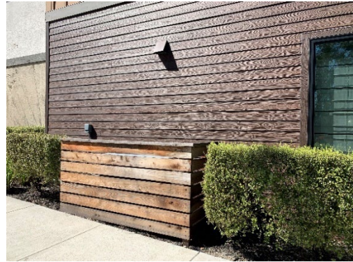
Screened mechanical equipment and vents painted the same color as the adjacent building facade.
